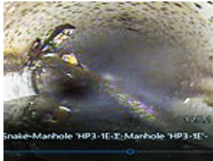
Cable protruding out of service line tap into mainline.
